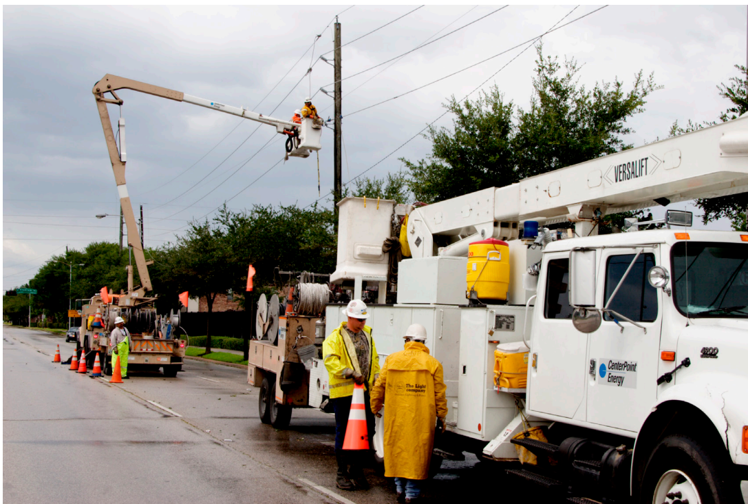
FIGURE 4-1 Center Point Energy personnel repair a downed power line (Houston, TX, September 23, 2005). Utility companies were out early to repair damage caused by Hurricane Rita. SOURCE: Ed Edahl, FEMA.
